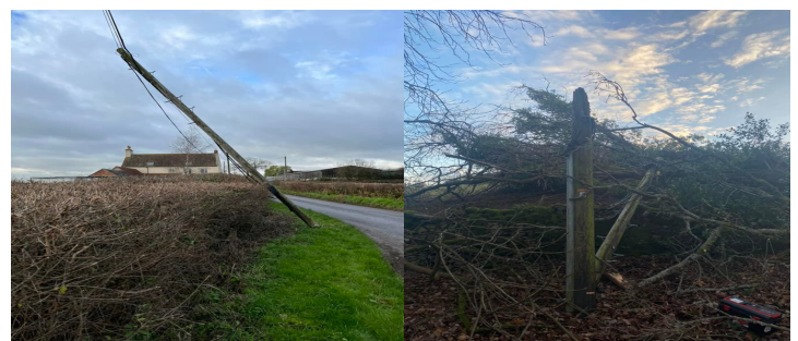
Top: the number of generators activated during Storm Arwen. Bottom: engineer photos of damaged overhead cables.
