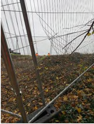
Damage to Heras fence
