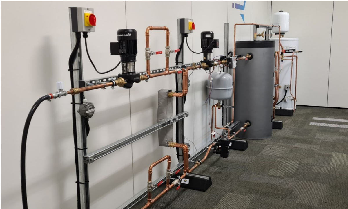
Heat recovery pilot system
