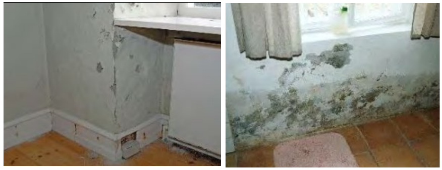
Figure 7 Paint and plaster deterioration (courtesy of Aalborg University)
